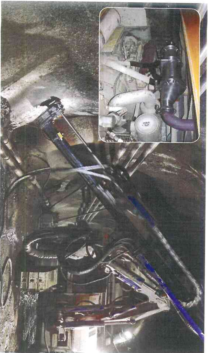
Airflow Catalyst Systems' EZ-series of converters, derived from technology developed and licensed by NASA, are used in the exhaust systems of underground diesel mining equipment to purge the air of potentially dangerous fumes. An EZ converter is installed for such an application (inset image).
